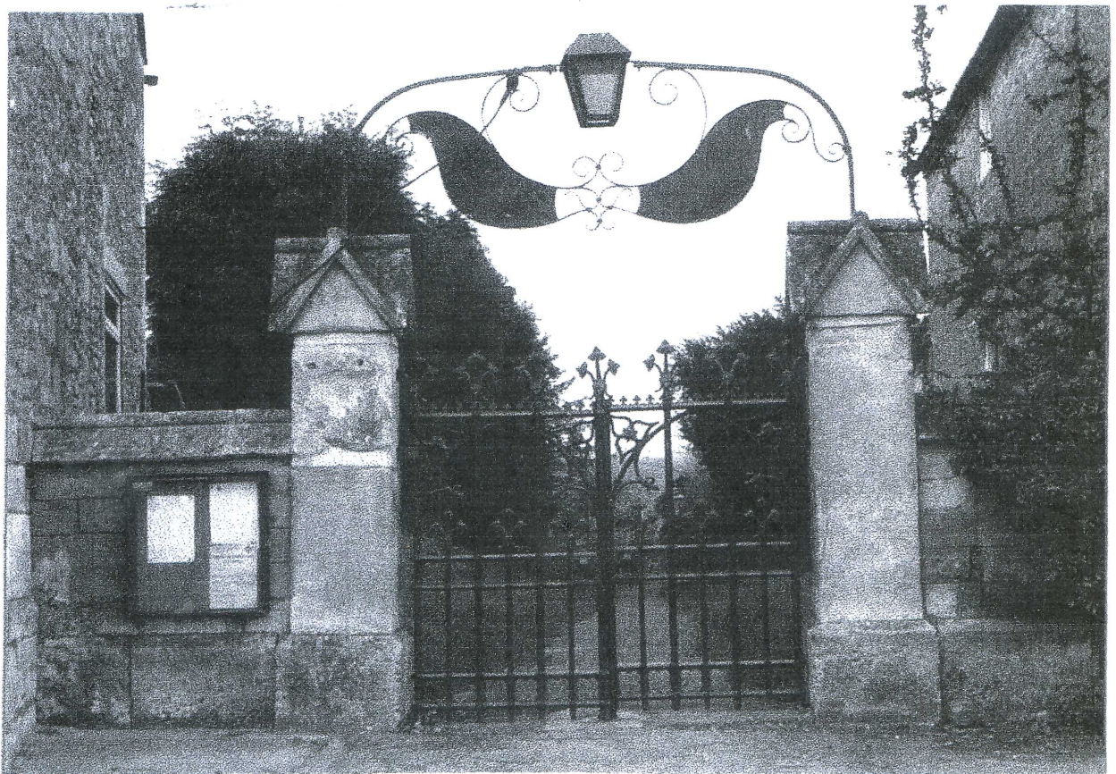
St. Paul's Church gateway needed urgent repairs to it's pillars in 1980.
