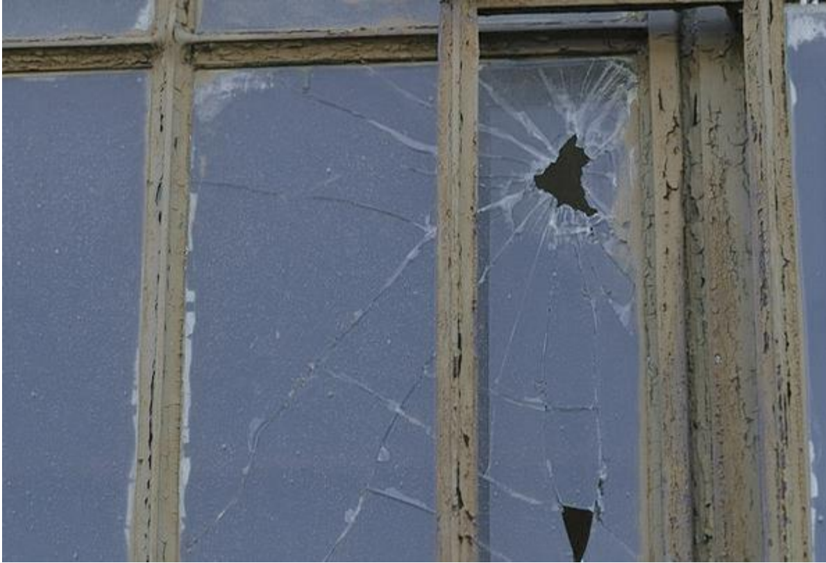
Gunshot damage to a window
